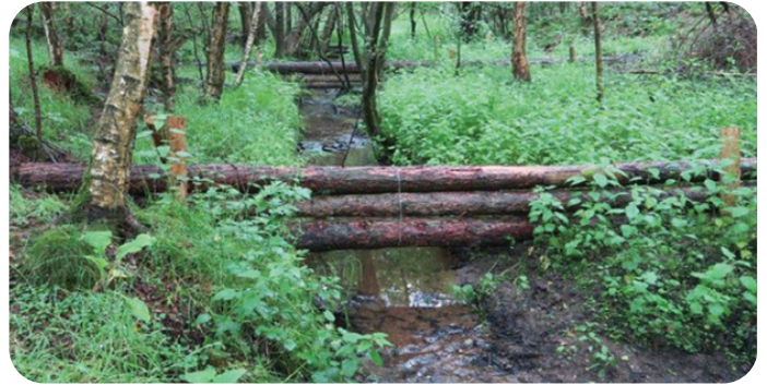
Leaky dam from the Designing and managing forests and woodlands to reduce flood risk: UK Forestry Standard Practice Guide
